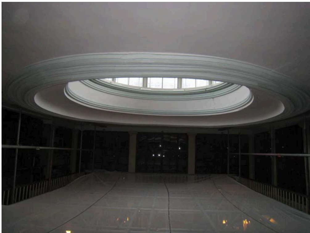
The dome is dropping into the library. The structure is currently supported by scaffolding, with netting to catch any falling debris.
