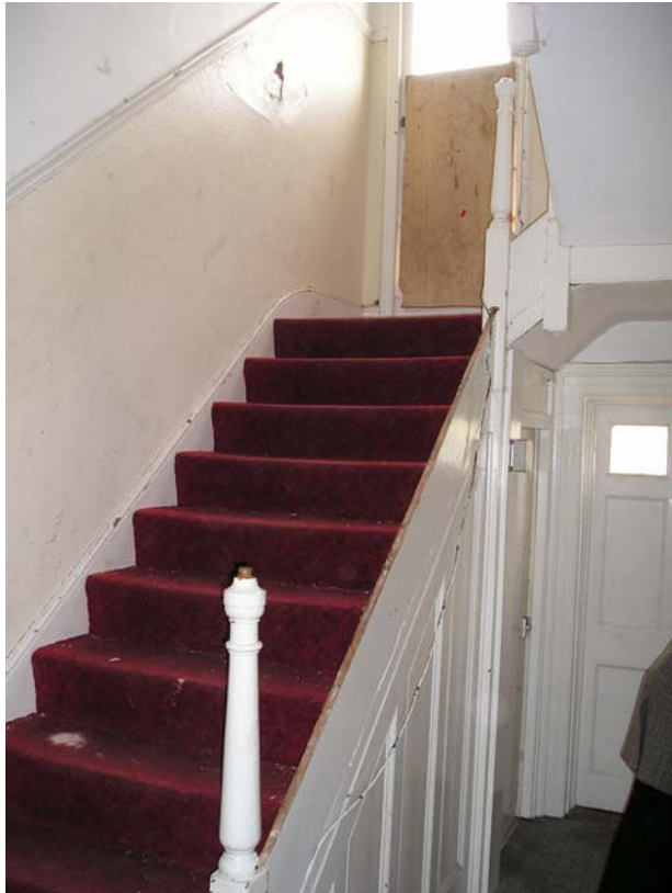
Hallway showing extensive damage to staircase
